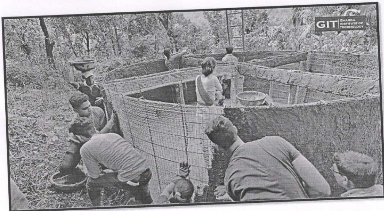
Application of Cement Concrete Mortar to the Outer periphery of the Water Tank
